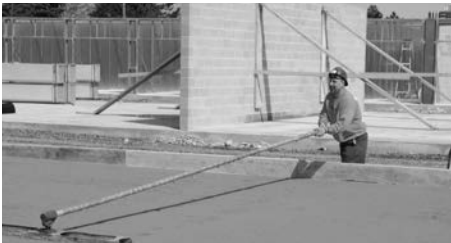
Used to consolidate surface voids and make a smooth surface for final finishing
