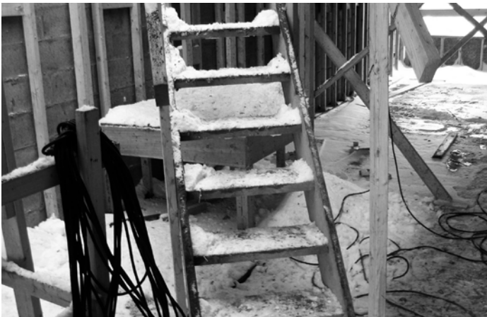
Figure 9-10: A fall hazard is caused by excessive ice and snow.
