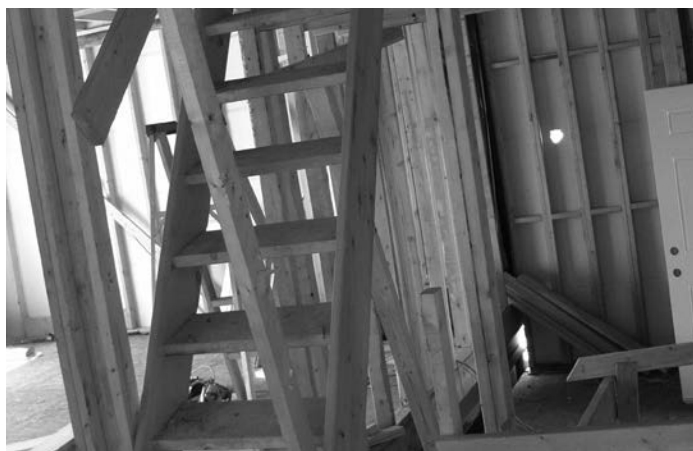
Figure 9-7: Slope of the stairway is steeper than the maximum allowed
