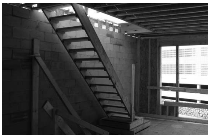
Figure 9-6: Stairway is too short and installed above a floor opening
