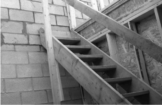
Figure 9-8: Stairway is poorly located
