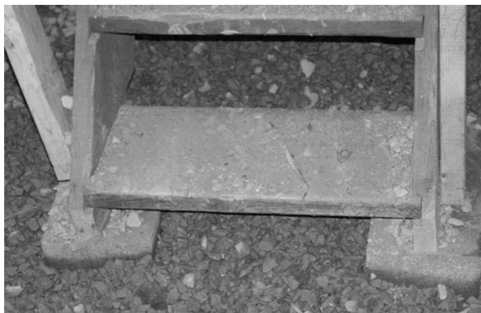
Figure 9-5: Bottom of stairway is not attached properly to the floor
