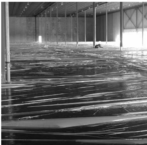
Used to harden the concrete surface. Wet curing covers such as polyethylene sheets are laid over new concrete
