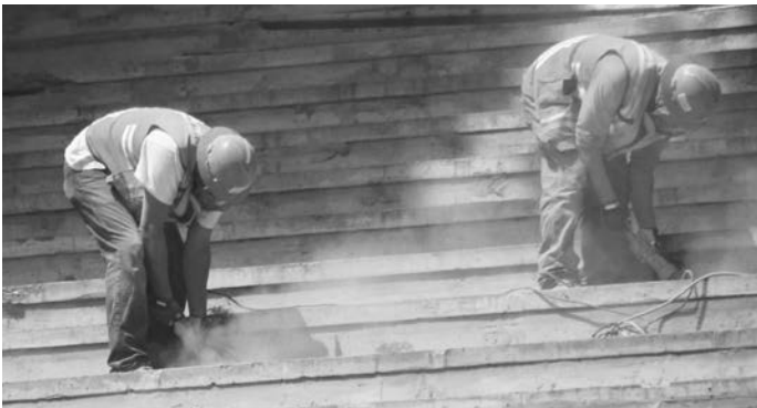
Figure 6-6: Silica Dust from Grinding Concrete
